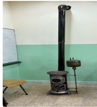
Figure 4. Photo of an unsafe heating system in an UNRWA - owned school in Syria
